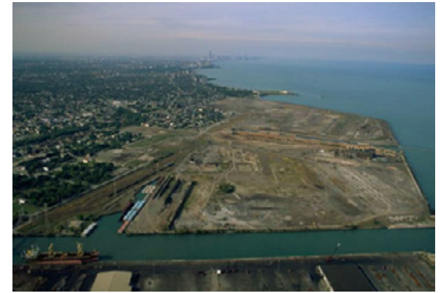
Alex MacLean, UIC Imagebase. US Steel South Works site in 1996 after demolition.
